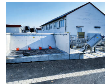
Sewer Sedimentation Reception Station – for collecting of sewers, gully waste and road sweepings
