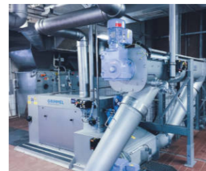
Conveyor – for screenings, sludge and grit to link various equipment modules
