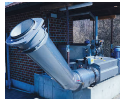
Sludge Receiving Station – as system solution with a Flat-Fine Screen
